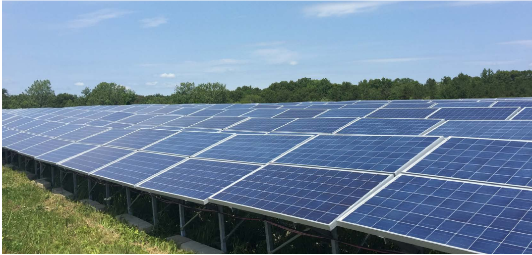
Concord's generation capacity includes this solar facility on an old landfill, which generates up to 1.7 megawatts of electricity. A second large array in town can generate 4.5 megawatts.
